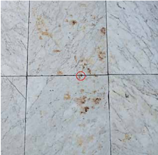
Figure 1. Stains from the floor in the staircase of the Staszic Palace. Test stain marked with a red circle
