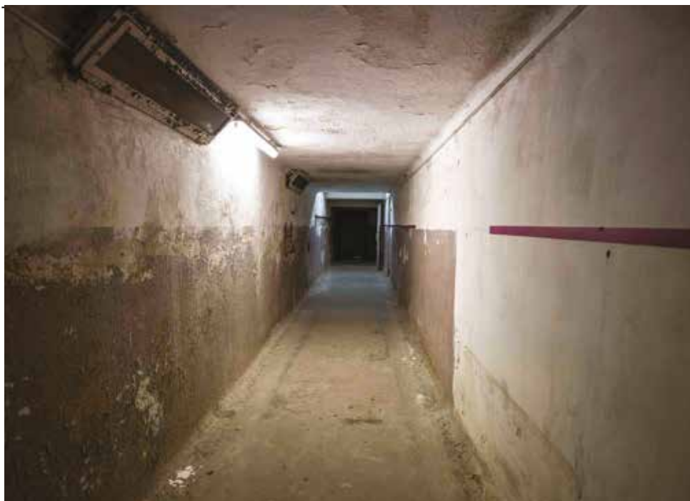
The underground corridor connecting Block X and the "Palace of Miracles". Photo Katarzyna Adamów (2023)
